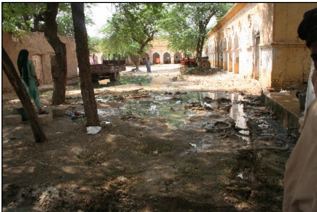
A school building in Sibi district, Balochistan after the water receded from the area.
